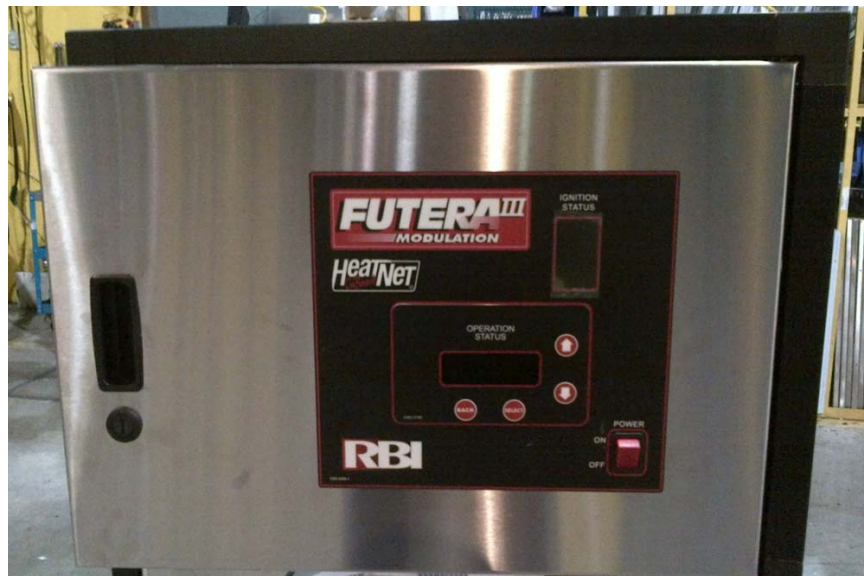
Figure5: HeatNet Control Panel Door
